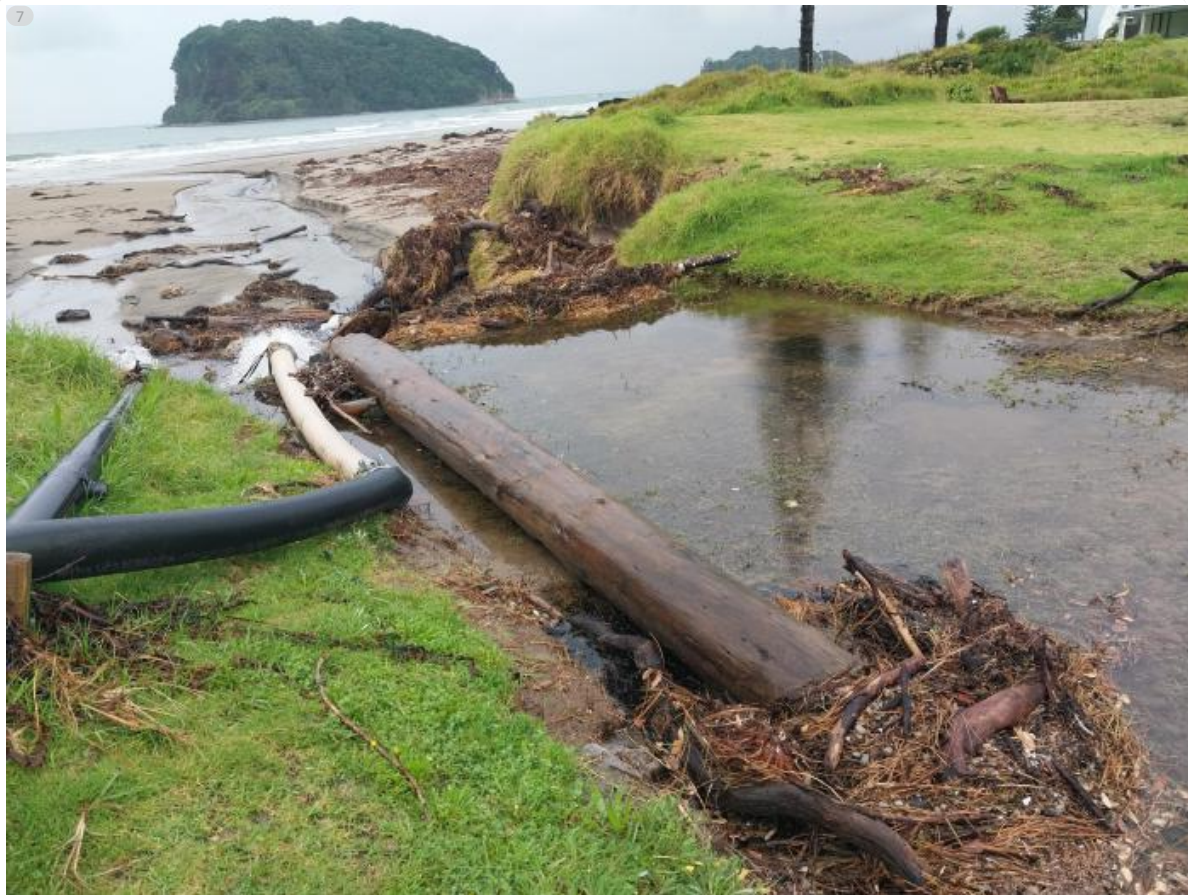
124 King Tides breach weir 20230227_105746.jpg
