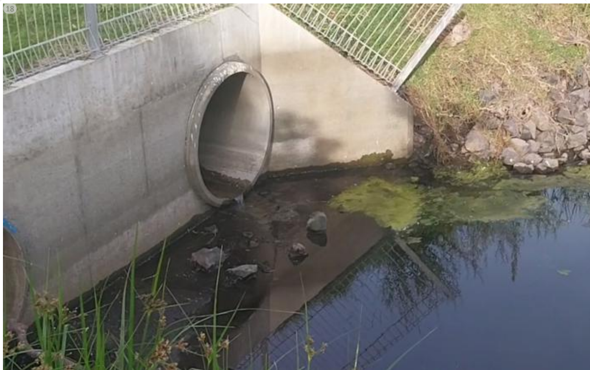
172 Discharge flow rate minor 20231205_000348_SC_.jpg
