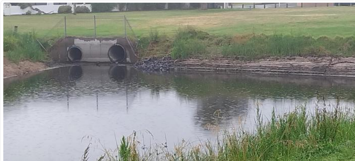
163 water table bleed tracks 20231118_085403.jpg
