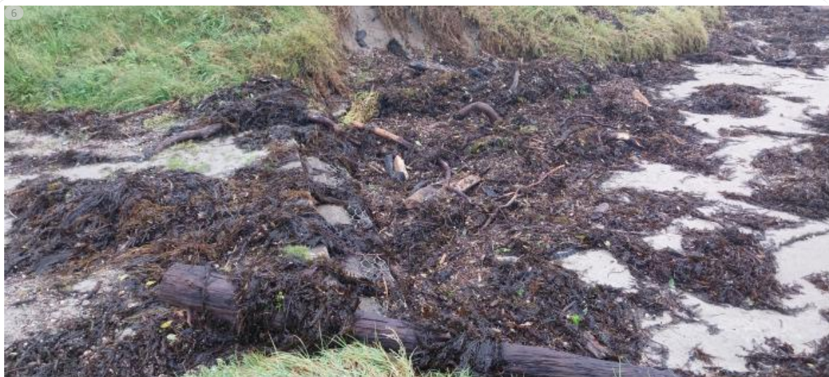
110 Weir after King Tides 1 November.jpg
