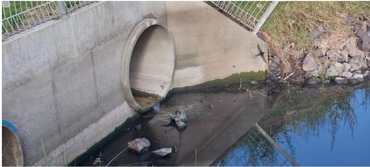
171 Discharge pipe flow rate small 20231116_081130.jpg
