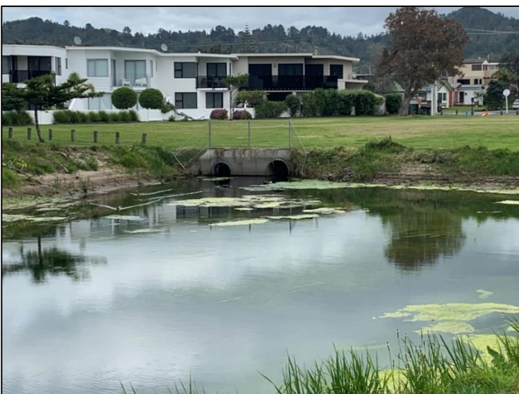
Figure 3: Two inlet pipes to the pond
