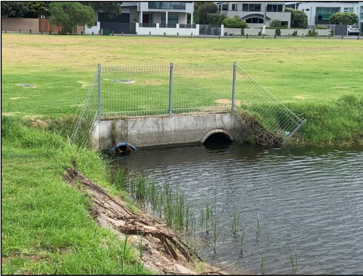
Figure 2: Inlet pipes to the pond during periods of sustained rainfall
