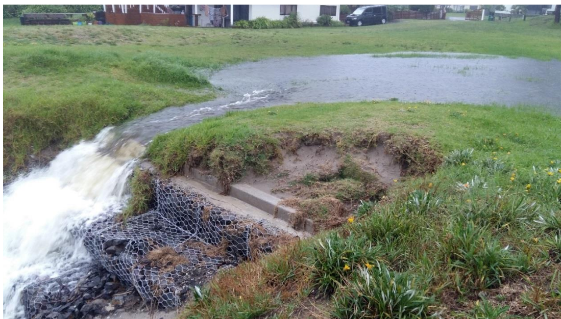
Figure 3 Williamson Park Pond Spillway with sediment build-up, overflowing 5 April 2017.
