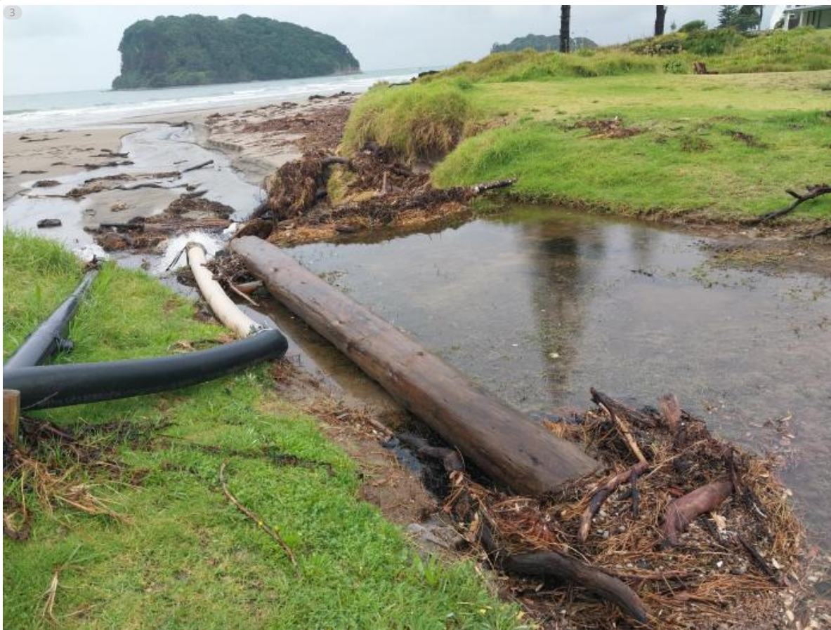
124 King Tides breach weir 20230227_105746.jpg
