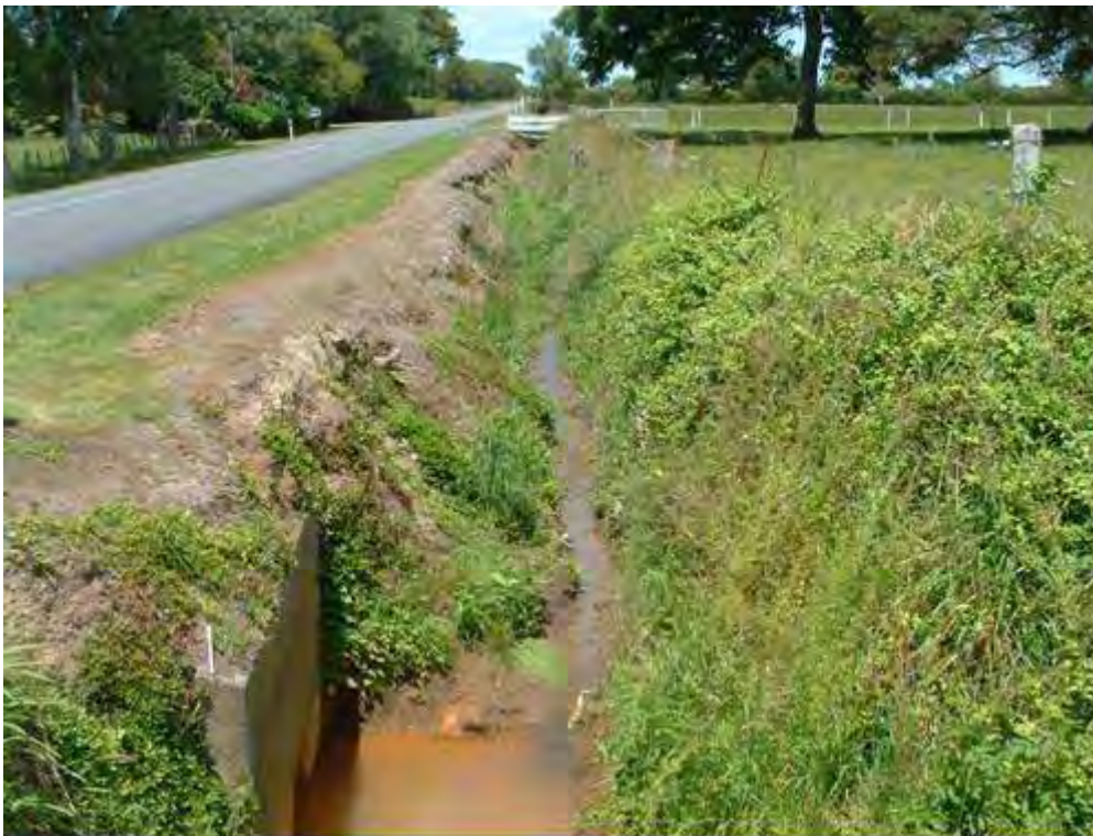
Photo 9 Bank erosion resulting from spraying the drain edge. The proximity of the waterway to the road will result in storm water runoff and pollutants directly entering the waterway
