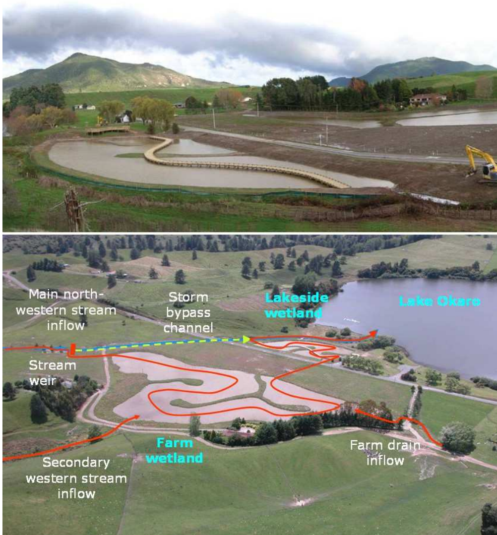
Figure 5-7: The constructed wetland at Lake Okaro at the time of construction. Top: Public access to the wetland is provided by a viewing walkway through the part of the wetland in the lake domain. Bottom: The stream water is forced to follow a convoluted flow path by the use of ridges within the wetland. The broken line indicates the short circuit path for flood events. [Photos and overlay: John Quinn, NIWA].
