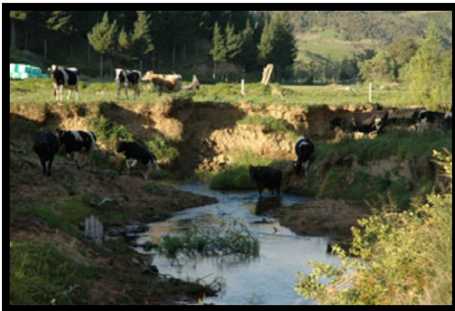
Figure 6. Slumping of the riverbank and stock access
