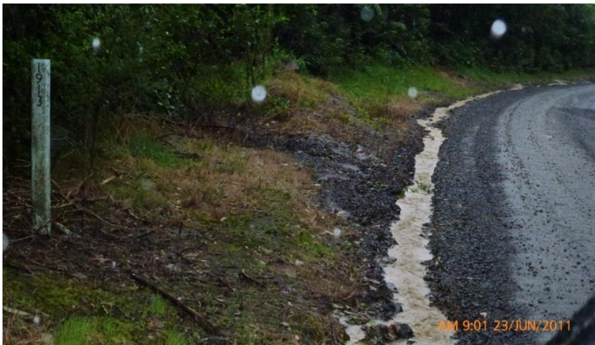
Figure 2: Storm water run-off missing cut out drain
