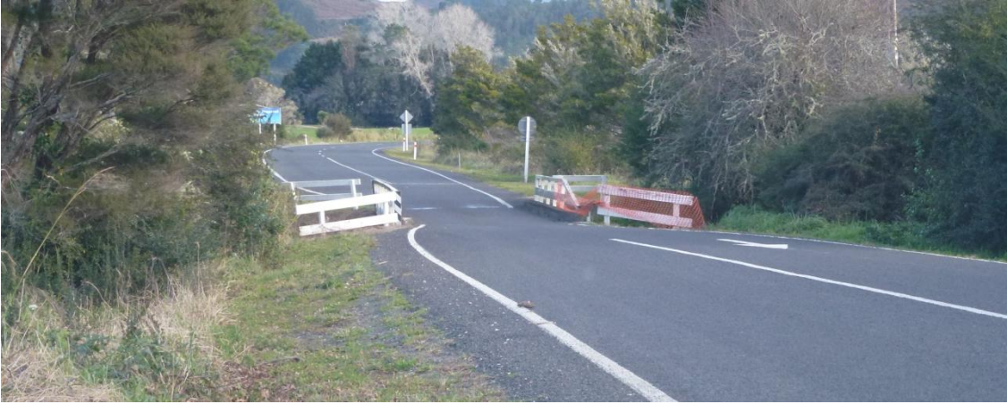
Figure 3: Bridge damage, Hot Water Beach Road
